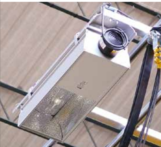
Crane light for bridge
