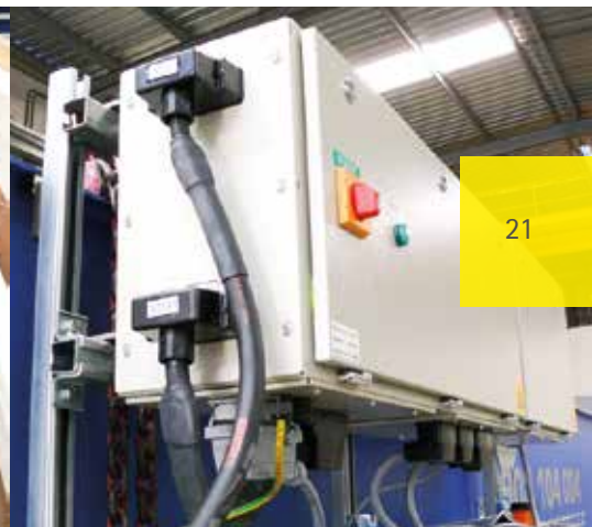
Bridge panel with plugs
